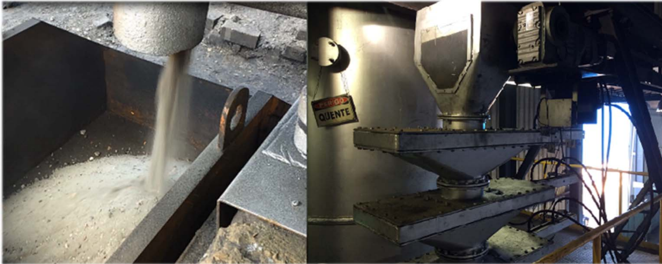
EXTRACTION SYSTEM ASH AND FEEDING SYSTEM
